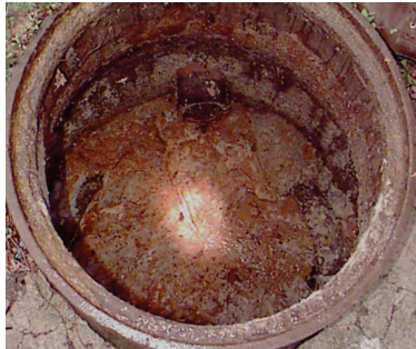
8 inch sanitary sewer blocked with FOG
