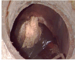
Grease buildup in sanitary sewer
