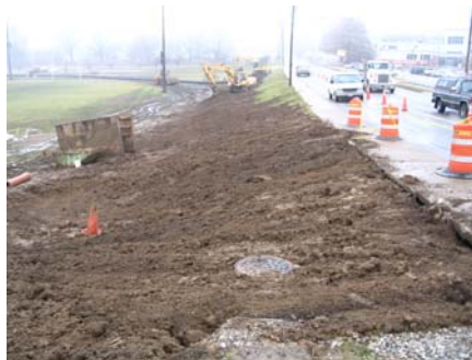
Replacement of the storm sewer on West 6 th Avenue required special construction in the wellfield.
