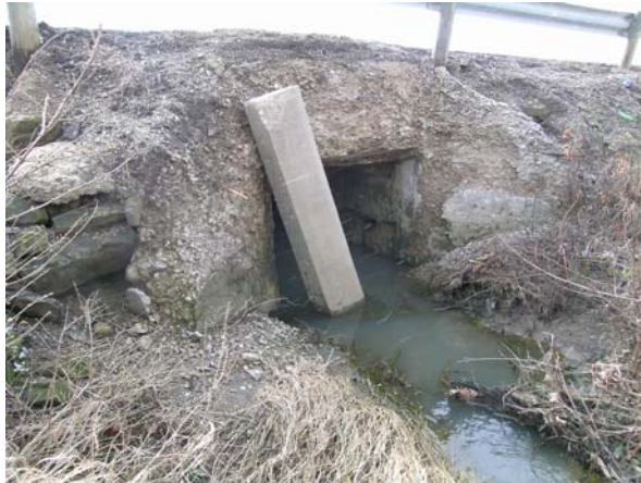
NCOL 6 Before Note the fallen headwall and edge of pavement
